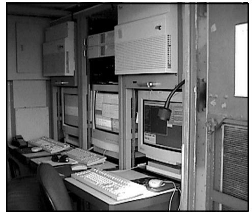
This PSTS operator’s station was demonstrated during exercises in Korea.
